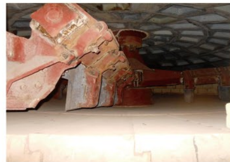
炉内件 Furnace inner parts
