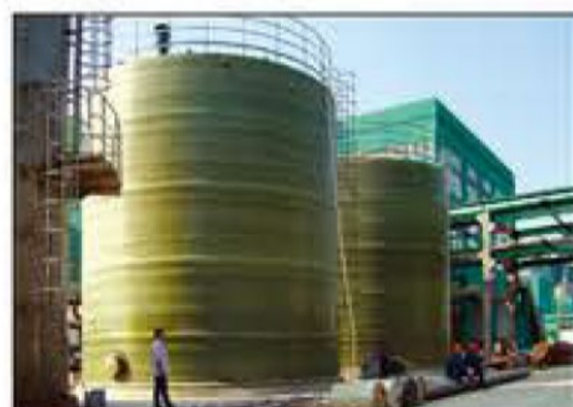
玻璃钢沉降罐 FRP sedimentation tank
