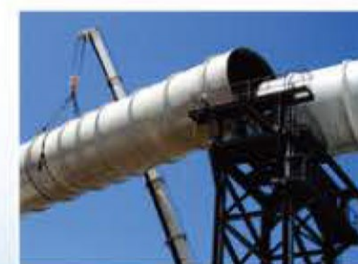
山东滨州热电厂烟塔合一工程 Fume pipe and tower syncretic project in Binzhou thermal power plant
