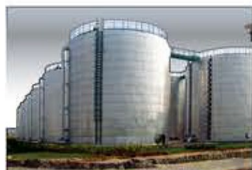
海水淡化大罐 Seawater desalination max tank
