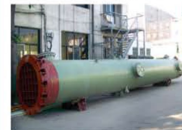
洗涤塔 Scrubbing tower
