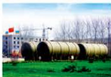
反冲洗滤液贮罐 back flush filtrate tank
